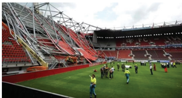
Fig. 3. Collapse of part of the roof at De Grolsch Veste stadium, Enschede, Netherlands, 07.07.2011 6
