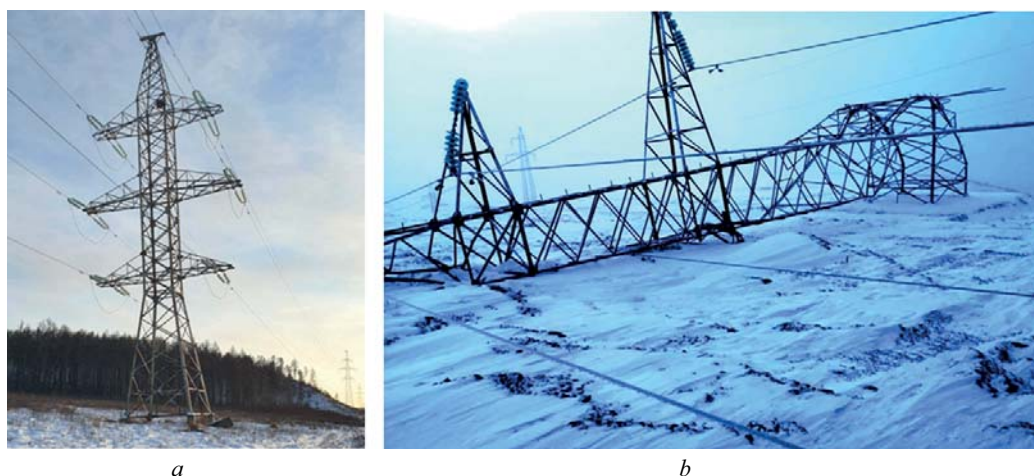
Fig. 2. Examples of damage and failures in power line structures: a — pre-failure tilt of an U220-1 anchor-corner support caused by frost heave of the foundations due to unanticipated freezing of the subsoil (Transbaikal region, December 2022); b — one of two fallen intermediate single-chain supports of type 2P220-1-6.8 due to wind loads exceeding design values (Irkutsk Region, Nov 2019)
