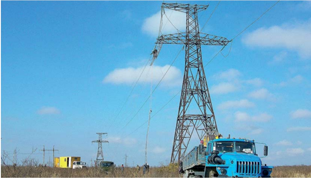
Fig. 3. Reconstruction of the 220 kV “Afipskaya – Krymskaya” overhead line, involving the replacement of old ASO-300 conductors with high-temperature GTACSR 217/49 conductors manufactured by the Japanese company J-Power Systems, using modern “tension-assisted installation” technology [12]
