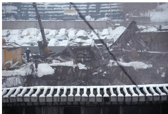
Fig. 2. Collapse of coverage at the market of Basmanniy State Unitary Enterprise, Moscow, 23.02.2006 5
